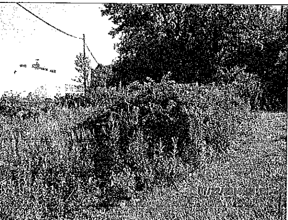
Description: Looking at riprap swale at northwest corner of proposed building addition.
