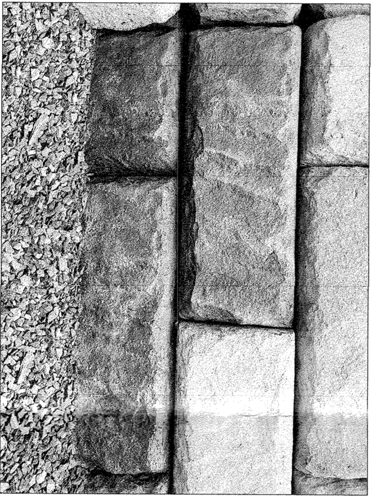
9 PHOTO 9 STAINED LIMESTONE FACE CLOSEUP
