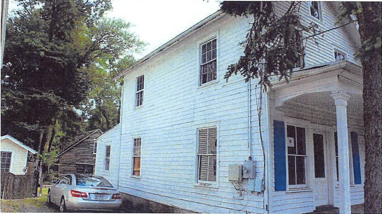
Will copy windows here with new simulated divided light windows. Note the inconsistent grill patterns of 2/2 (Victorian) and 6/6 (Colonial). We will present three options, one as is, one with 2/2 at first floor and 6/6 at second (like front has), and one with all 6/6 lites.
