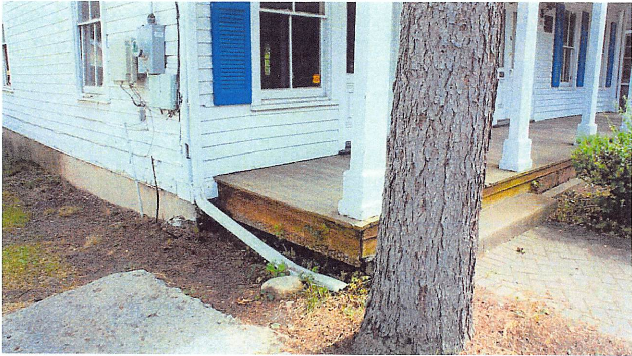
Cement Parging over bulging stone foundation at left (east) wall. Note inconsistent clapboard width from original front wall. We propose to rebuild this wall with concrete and use salvaged stone to build a new stone veneer wall to mimic what was originally there. We also propose to rebuild the wall and use 4" clapboard to match the front elevation.
