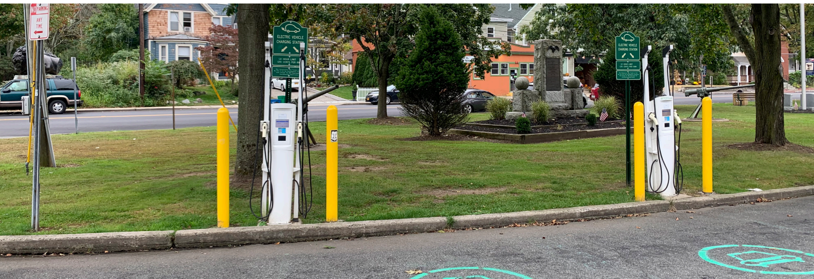
EV charging stations in a Sparkill parking lot © MUD Workshop
