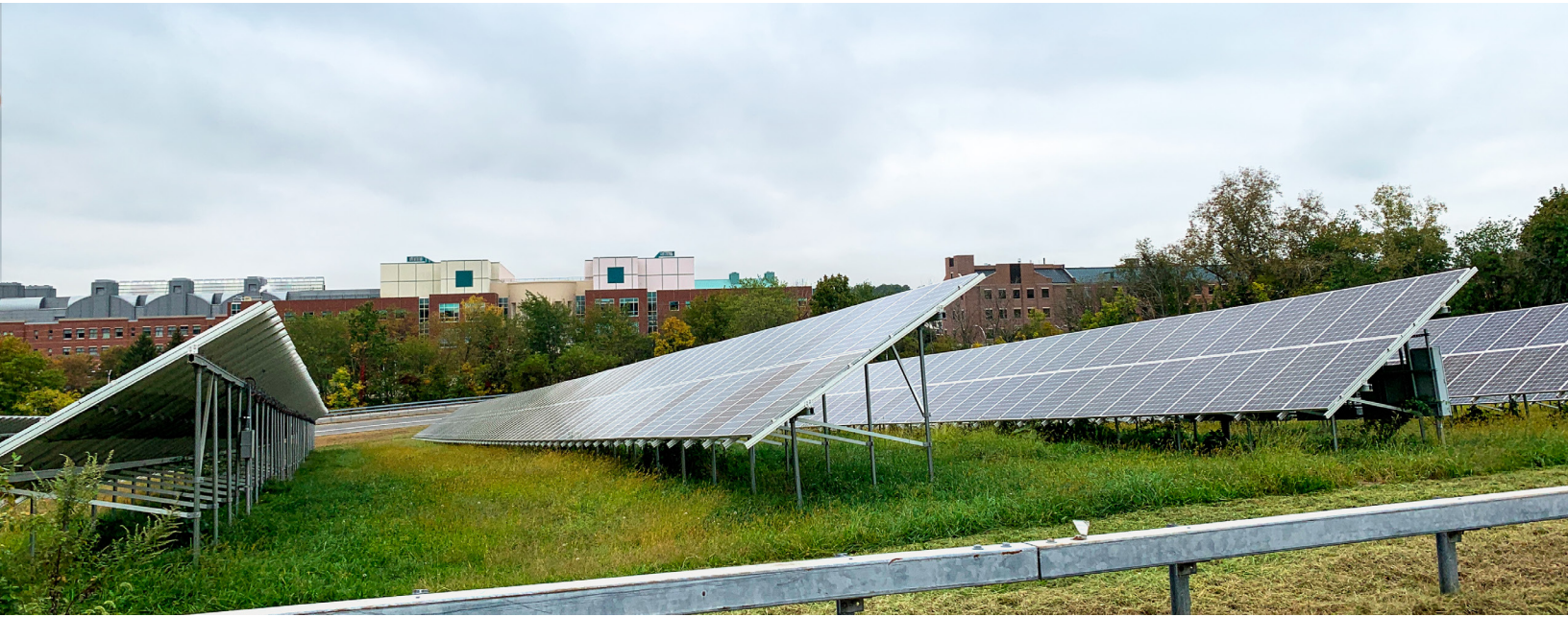
Solar panels at the North Middletown Road and NYS Route 304 interchange, Pearl River © AKRF
