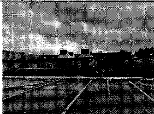
Description: Standing north of existing building to be removed on #125, looking south at area of new building expansion.
